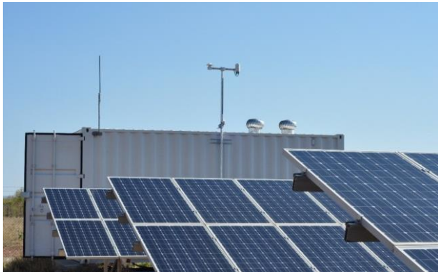
Figure 1: CloudCAM installed at Epuron's Kalkaringi high penetration solar power station in central Australia
