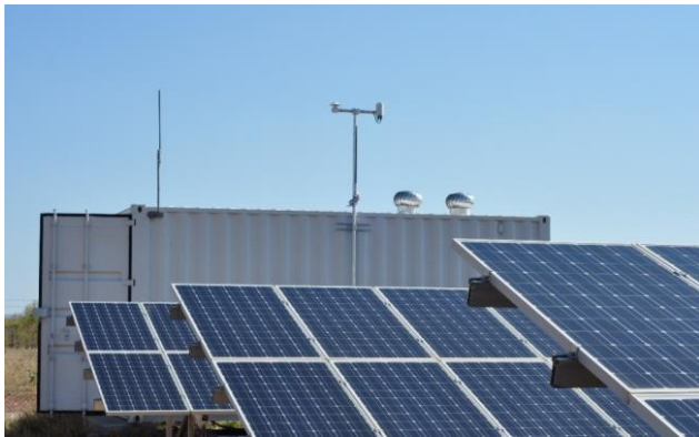
Figure 1: CloudCAM installed at Epuron's Kalkarinaji high penetration solar power station in central Australia
