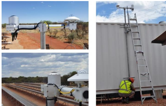
Figure 1: Fulcrum3D CloudCAM & Kipp & Zonen SMP11 pyranometer at Ti-Tree, NT. Installation and integration completed by Fulcrum 3D's in-house technicians and engineers.
